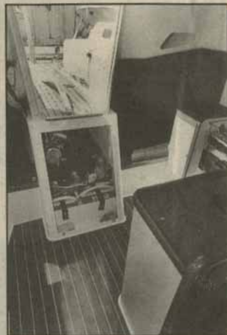
The engine installation is very neat, access being from either under the companionway or from the quarterberths.
